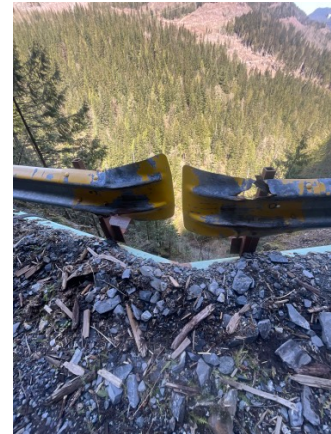
Guard rail damage
