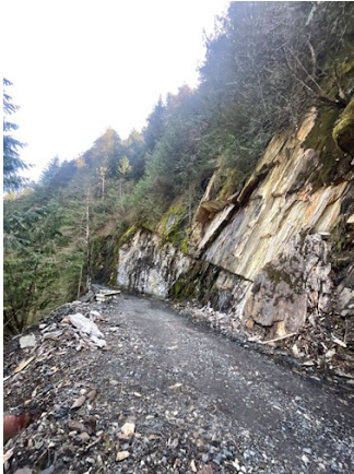
Approach from town and recent rock fall
